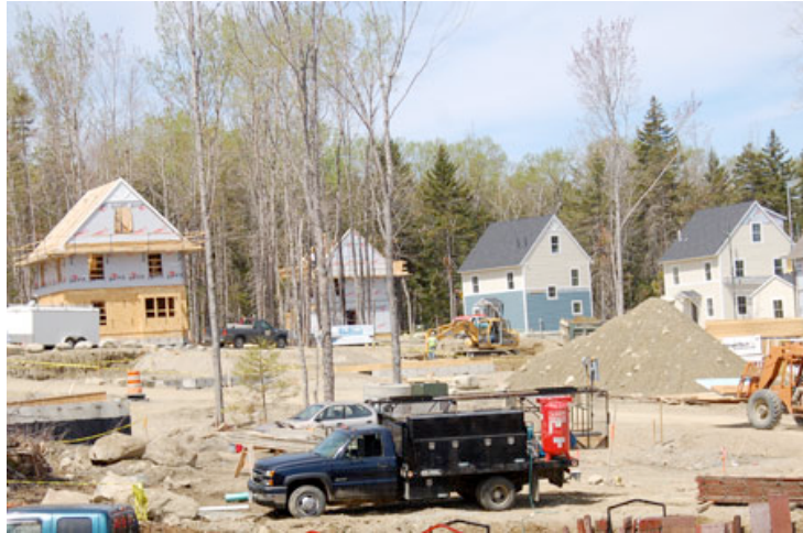
Several more foundations, now under construction, will complete this section of "walk-to" houses, one part of the Northeast Creek Neighborhood being developed by the Bar Harbor Housing Authority.—ROBERT LEVIN PHOTO
