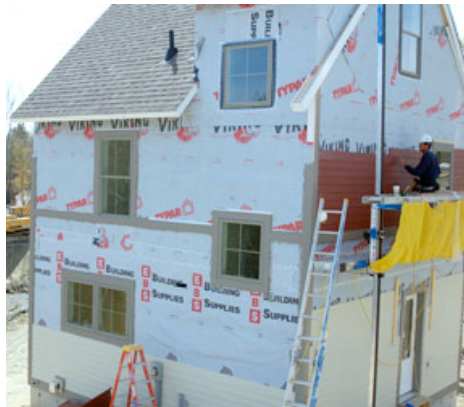
A worker for Bowman Brothers Construction installs cement board siding on a house at the Northeast Creek Neighborhood recently. Cement board is a more expensive, but more environmentally-friendly option than vinyl siding.—ROBERT LEVIN PHOTO
